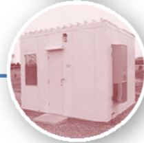
Substation Control House
